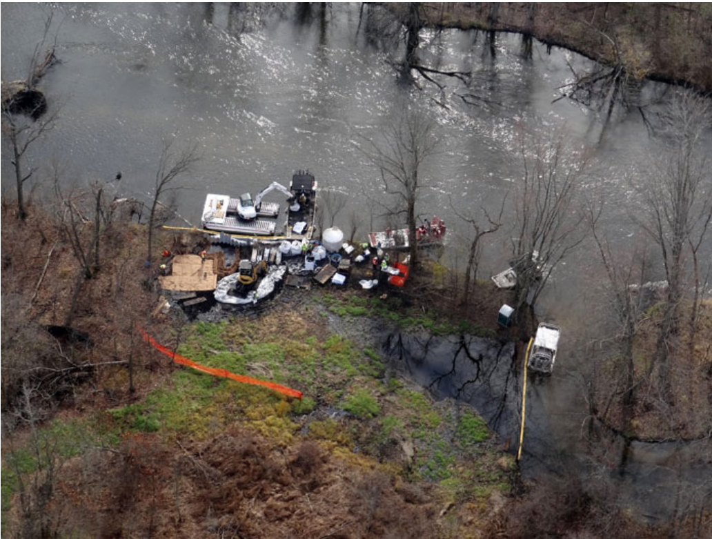
Excavation of oil-contaminated soil from the overbank area located at MP 11.01 (11/15/2011) (EPA)
