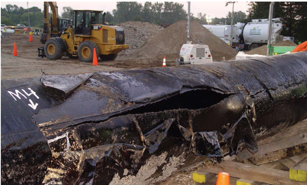
The ruptured pipeline after it was excavated AP Photo/National Transportation Safety Board
